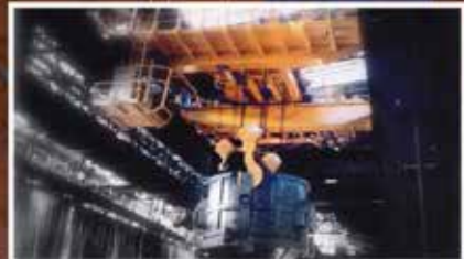
100/16 TONN. CASTING CRANE
