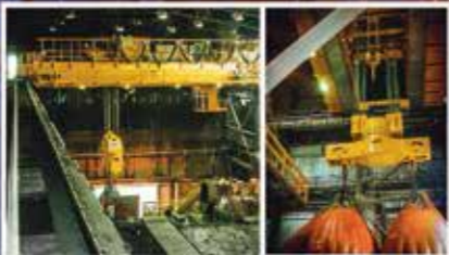
130/40/8 TONN. ROTATING BLOCK CASTING CRANE
